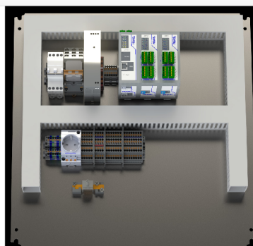
Fig. 3 – Internal arrangement: PLC, relay-output modules, circuit breakers, phase selector, PSU and I/O terminals on DIN rail
